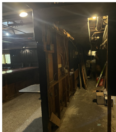
Electric/HVAC behind bar
